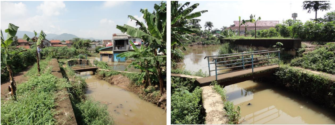
Figure 2.12: End of flood wall near Cieunteung with the gate top level about 1 m lower (March 2016)
